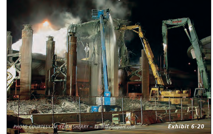
Demolition during the first phase of SR 519 project. Photo courtesy of WSDOT.
