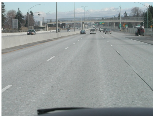
Figure A3.1. Studded Tire Wear on PCCP
