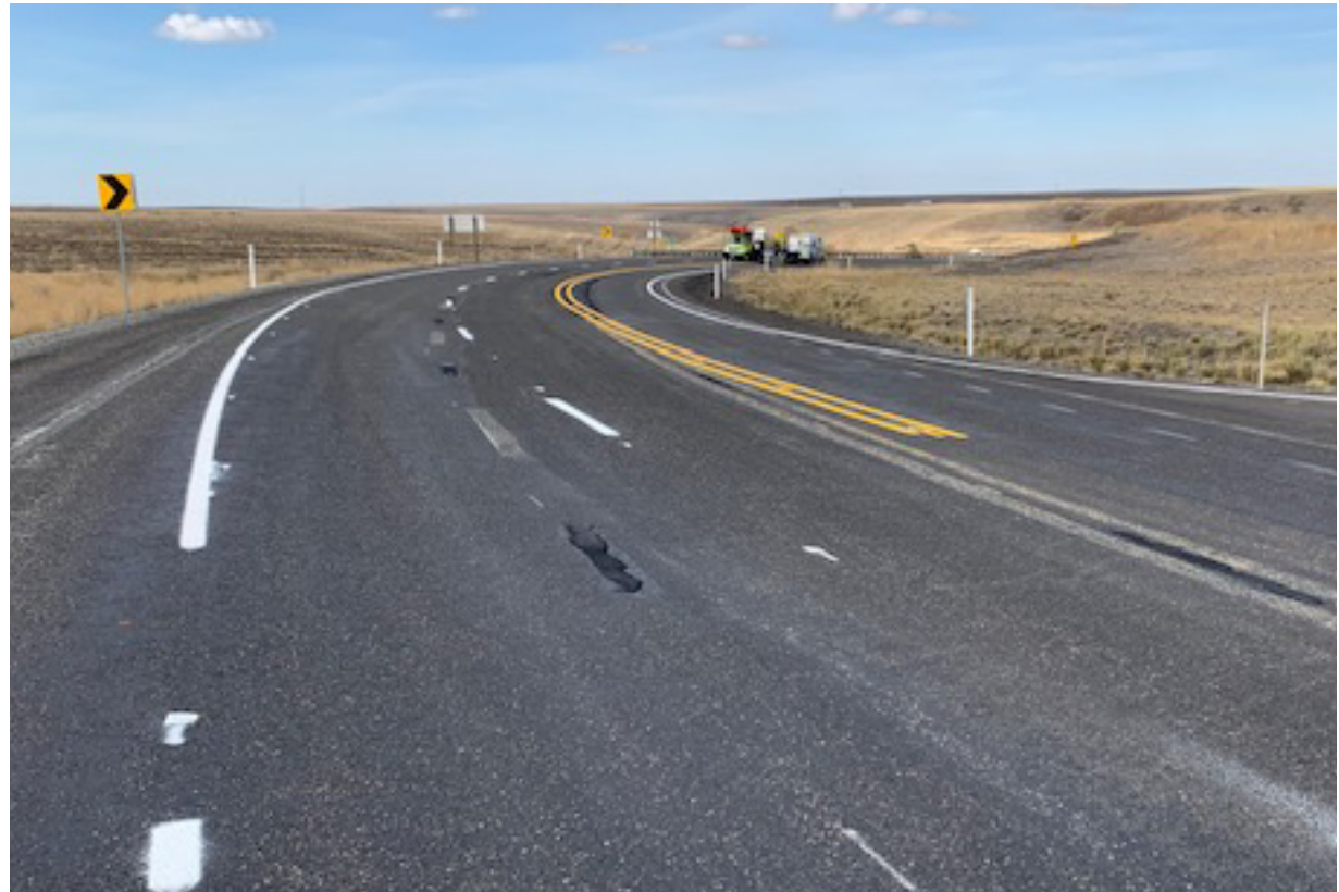
The compound curve has been smoothed out, reducing the likelihood of lane departures.
