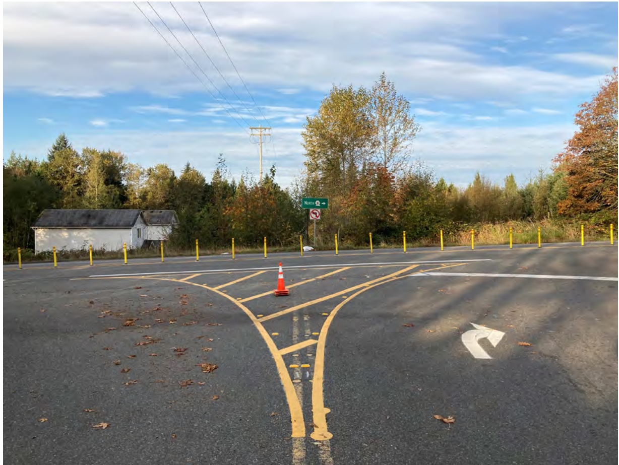
Pylons, striping, and signing to prevent left-hand turns from SR 9 to 60th.
