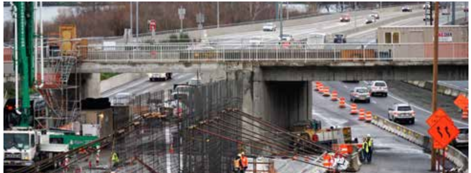
The $455 million SR 520 Montlake Project, now underway in Seattle, is a design-build project.
